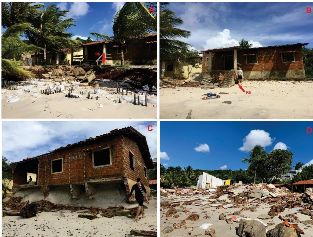
Figure 6. P7 Records of erosive processes in the region of profile P1. (A) Location of the reference level (RN) in July 2017; (B) Condition of the reference level in March 2018; (C) Foundation of the former residence on the backshore beginning to lose support in May 2018; and (D) Debris of the residence following continuous erosion.
